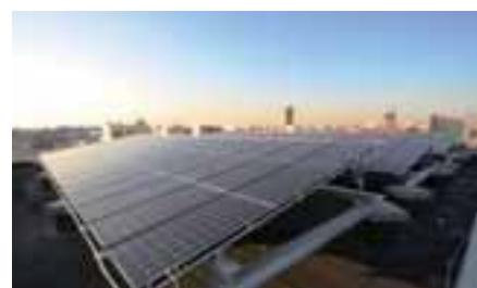
Photovoltaic power at Ukima site
